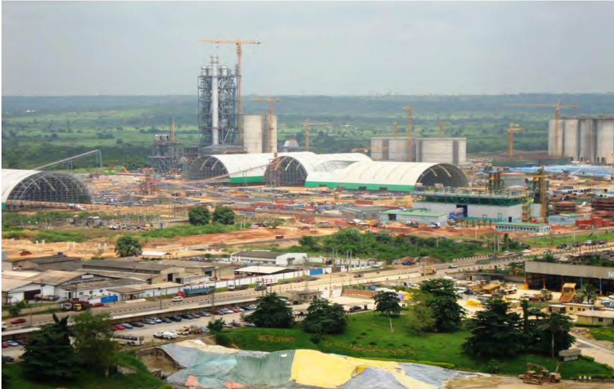
Figure 11: Aerial View of the Ewekoro II Plant - Showing material storages and kiln pre-heater standing
